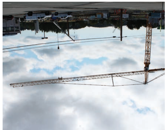
The 165-foot tower crane at the Clean Water Facility Project construction site.
