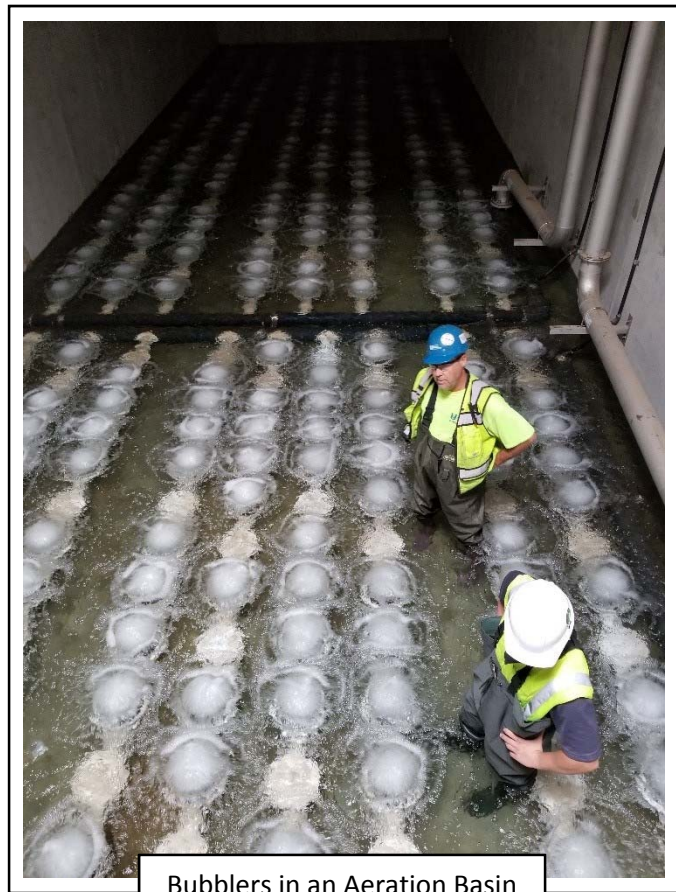
Bubblers in an Aeration Basin
