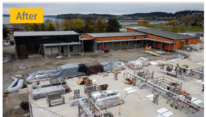
Look how far we've come! Before and after view of the maintenance and administration buildings at the new Oak Harbor Clean Water Facility.
