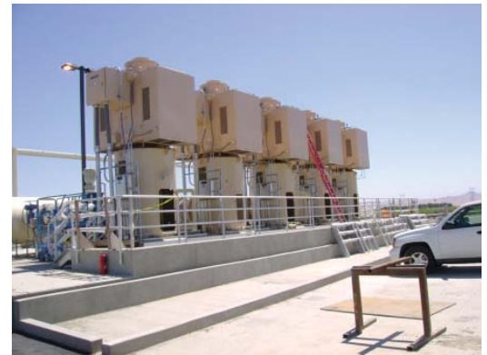
Provided detailed control system design for the intake pump station including 5-3,000 hp pump, the PLC and SCADA control system, programming services, and engineering services during construction.
