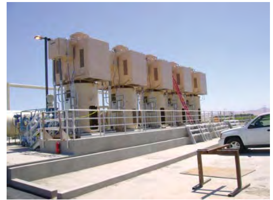
Provided detailed control system design for the intake pump station including 5-3,000 hp pump, the PLC and SCADA control system, programming services, and engineering services during construction.
