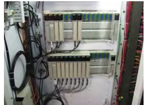
Carollo Engineers provided hardware, software, programming, and complete systems integration services.
