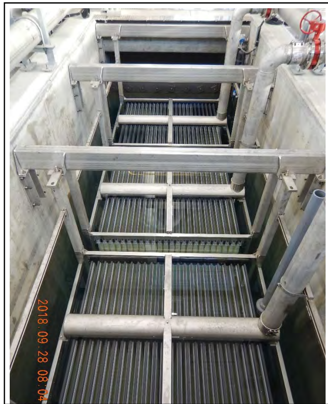
Membrane Cassettes submerged in Potable Water
